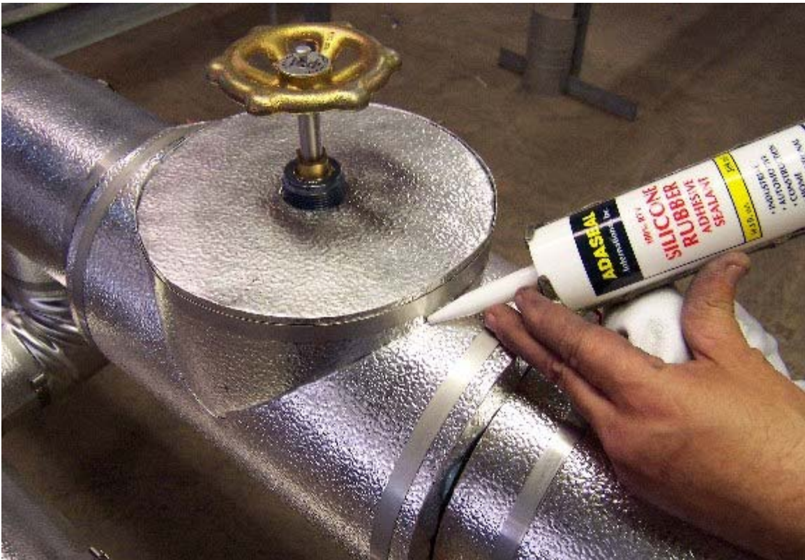
Aluminum cladding valve.
