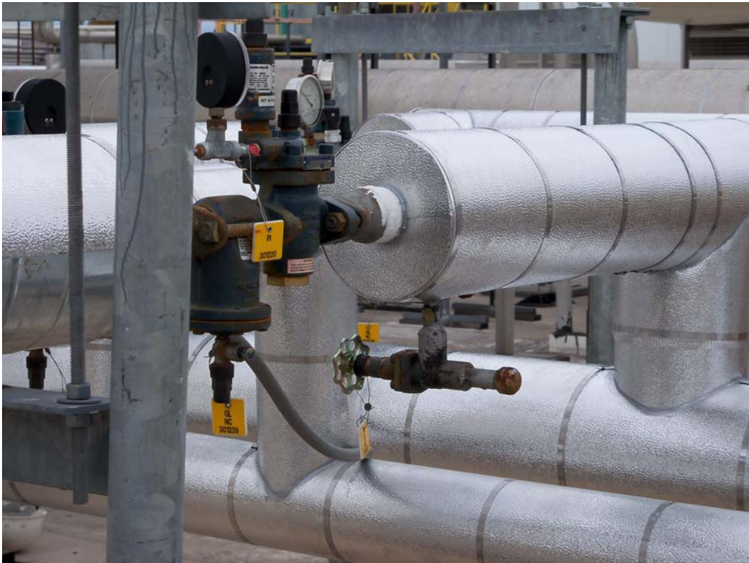
Aluminum cladding (transition to non-insulated line with cap).
