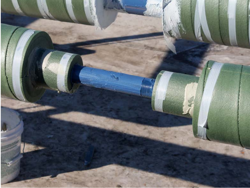
Double layer expansion joint assembly, 16" gap in 2 nd layer.
