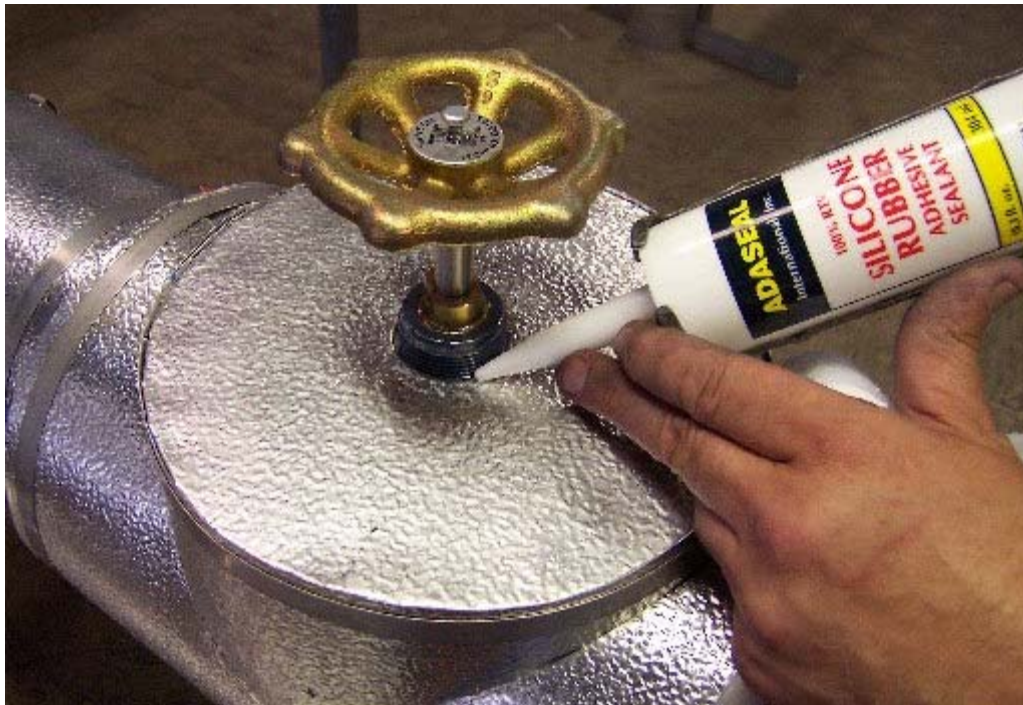
Aluminum cladding valve stem.
