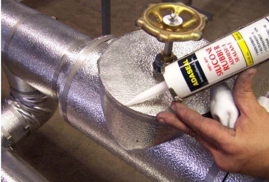
Aluminum cladding valve.
