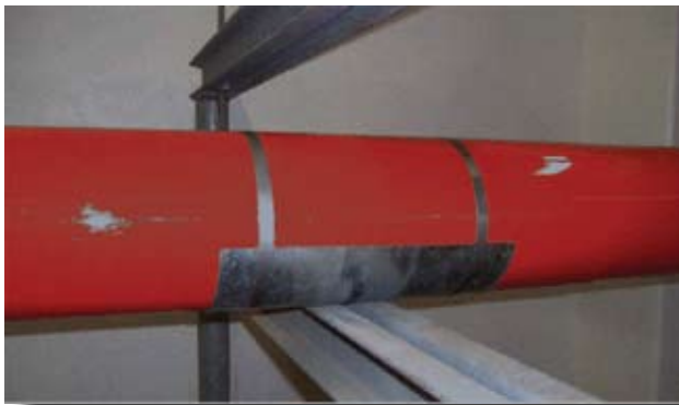
PVC (insulation protection saddle and banding).
